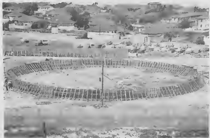
1 THE FRAME is up, the foundation is poured. All this took place after careful surveying and leveling of the site.
